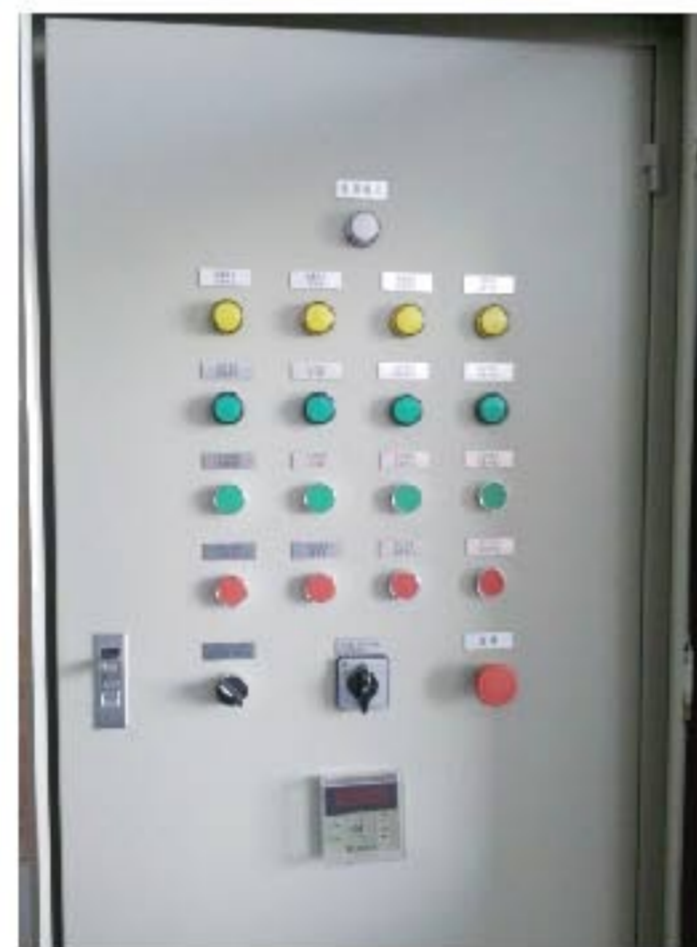
电控箱 Electric Cabinet
